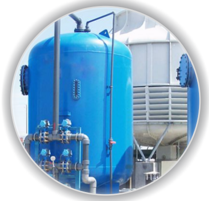
Carbon & Sand Filter
